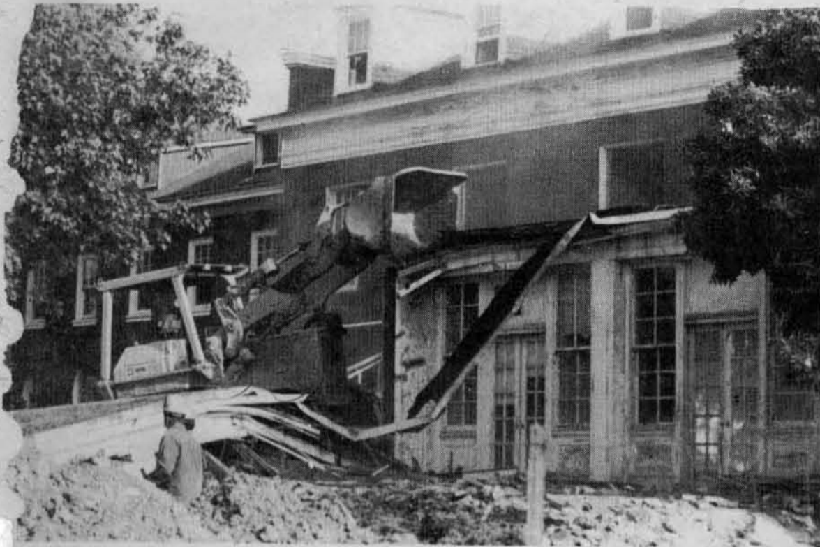
INSIDE OUT: The front part of the Old Administration building was the first to go. After a few days the only thing left is rubble [photo by Liz Kraft]
